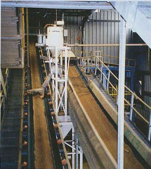
Air Transport System for Returning Collector Fines to Finished Belt
